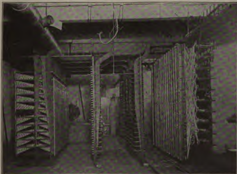
PART OF DISTRIBUTING RACKS IN REAR OF SWITCHBOARD.
